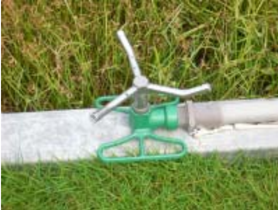
Figure 8. Water sprinkler for the green roof system.
